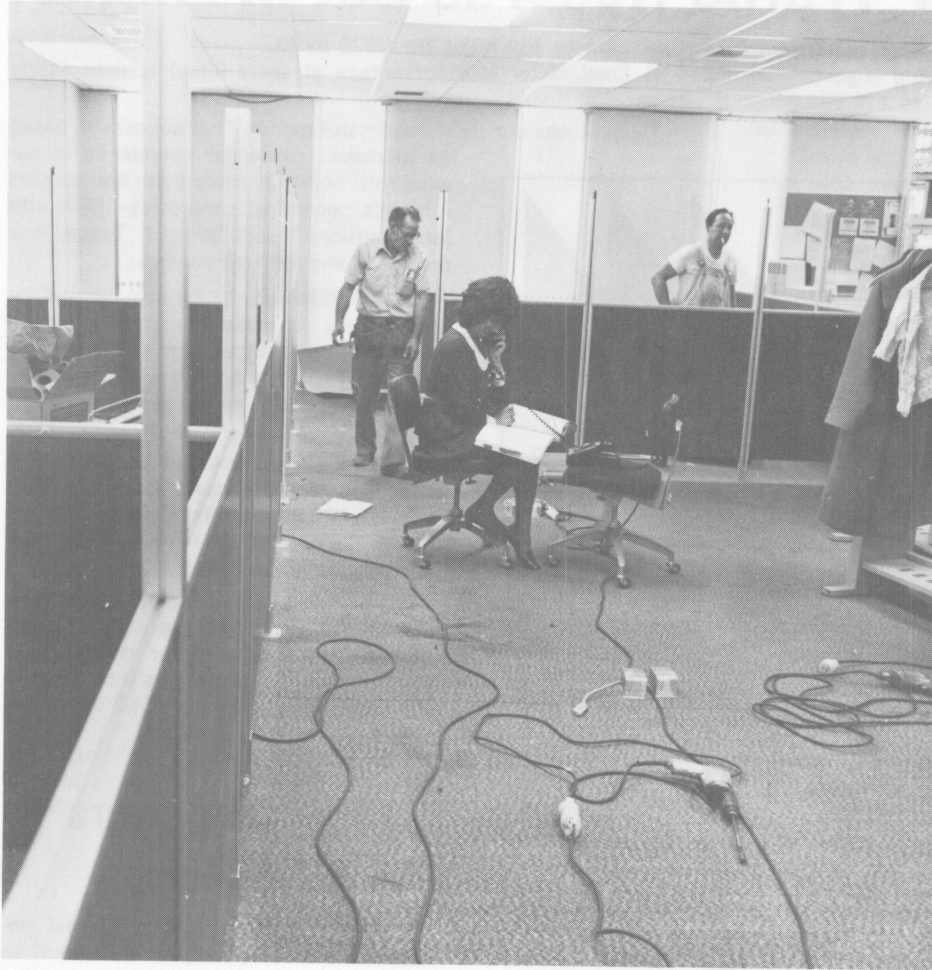
CONSTRUCTION CONFUSION —Annette DeNunzio, clerk in the accounting department, was temporarily without her desk while workmen constructed office cubicles for the purchasing department on the 9th floor of the Mills Building. Purchasing, which moved to San Mateo from Phoenix in August, occupies space formerly used by payroll and accounts payable.
